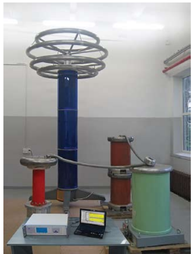
VA-3.1 Peak Voltmeter pictured as part of reference measurement bench. Picture was taken in Mars-Energo high voltage lab
